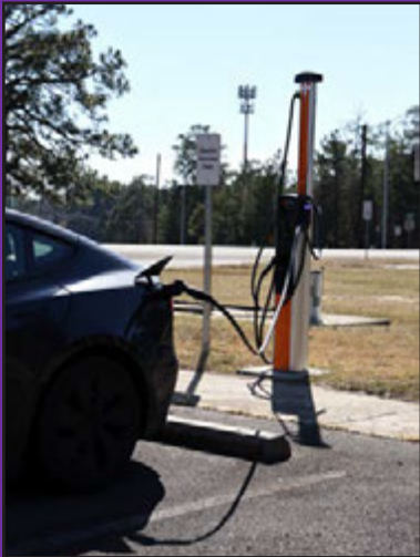
COVER PHOTO A vehicle charging at one of the new stations on Fort Polk. (U.S. Army photo by Angie Thorne)
