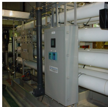
Reverse Osmosis Units
