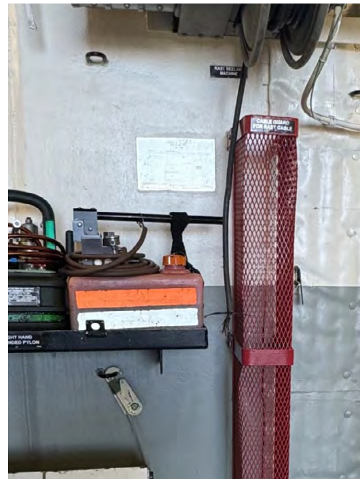
A broken electrical cable in the hangar bay of USS Nimitz (CVN 68) in the Pacific Ocean, April 4, 2025. (Courtesy photo by Lt. Cmdr. Ravi Patel)
