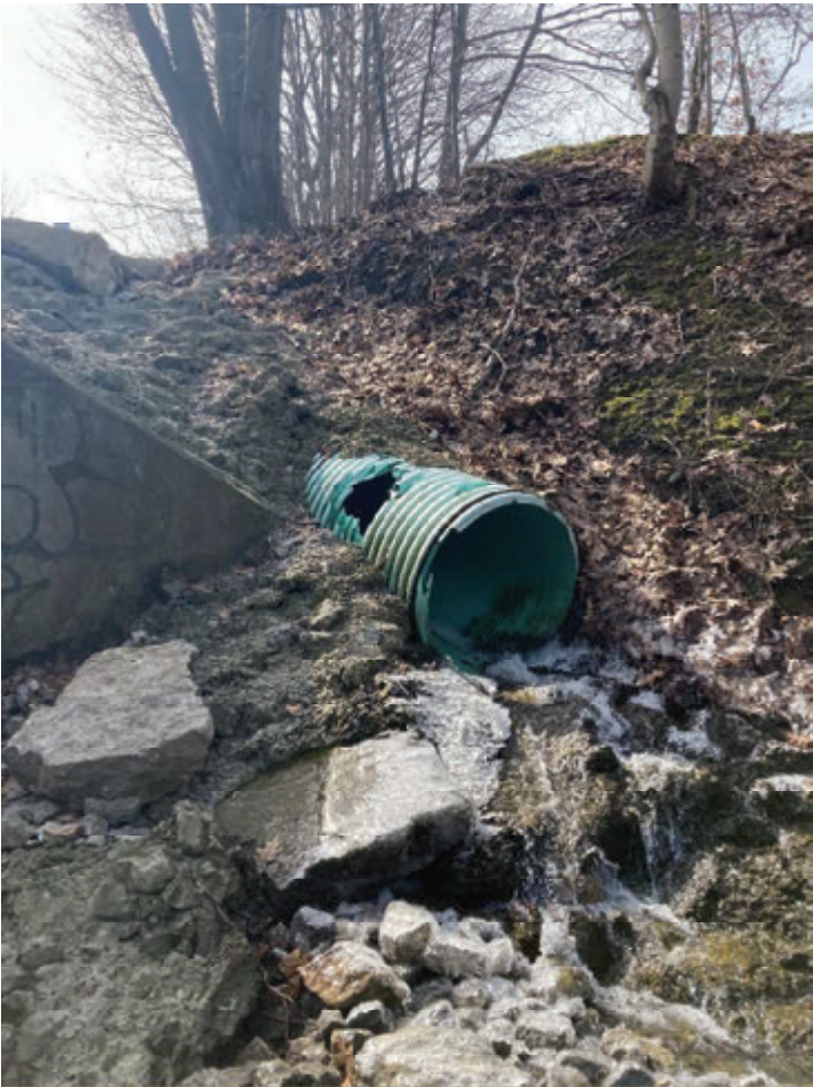
Photo 15: Effluent from culvert near Griffey Rd bridge
