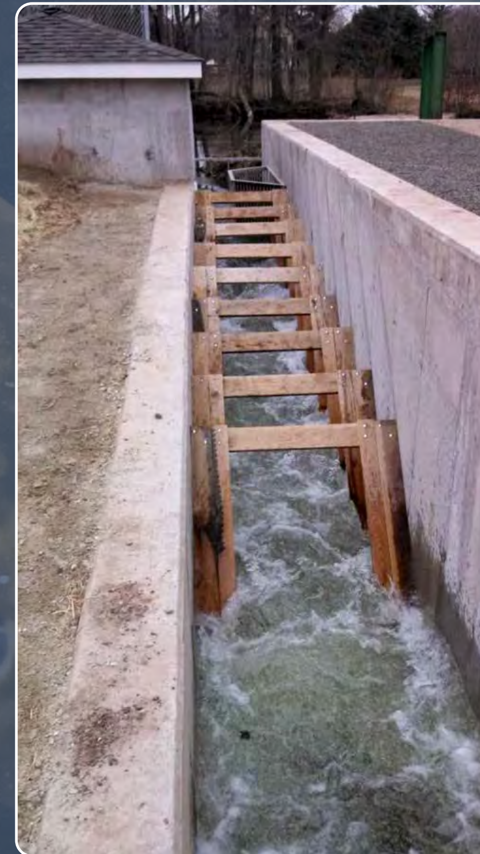
StanChem Dam Fishway on the Mattabesset River in East Berlin, CT (Source: The Connecticut River Salmon Assoc.)
