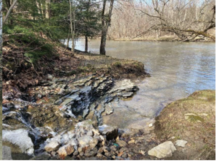
Photo 14: Effluent from culvert near Griffey Rd bridge
