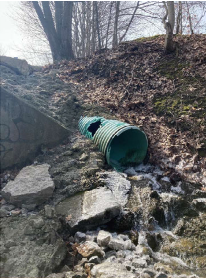
Photo 15: Effluent from culvert near Griffey Rd bridge
