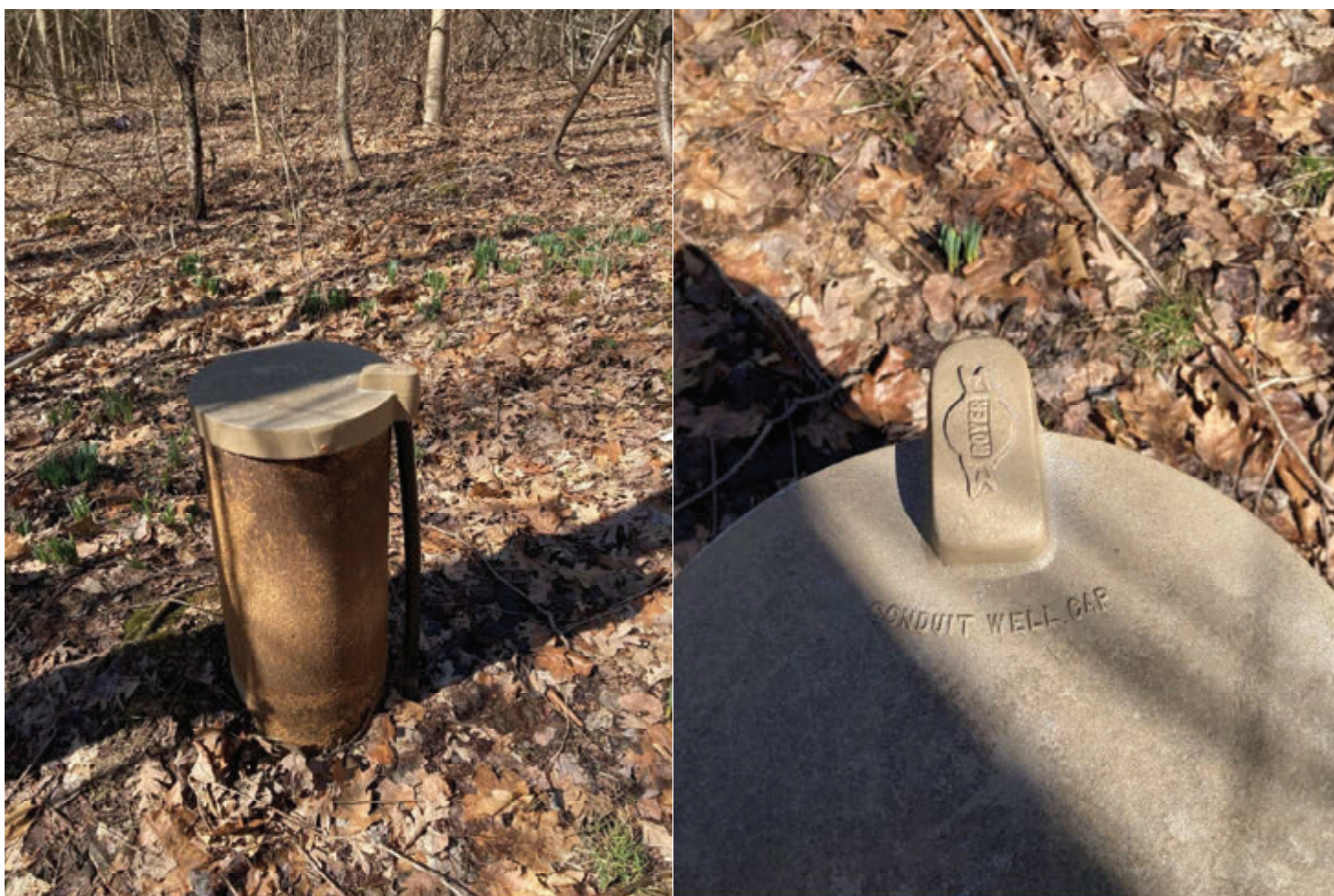
Photo 35: Steel well casing
