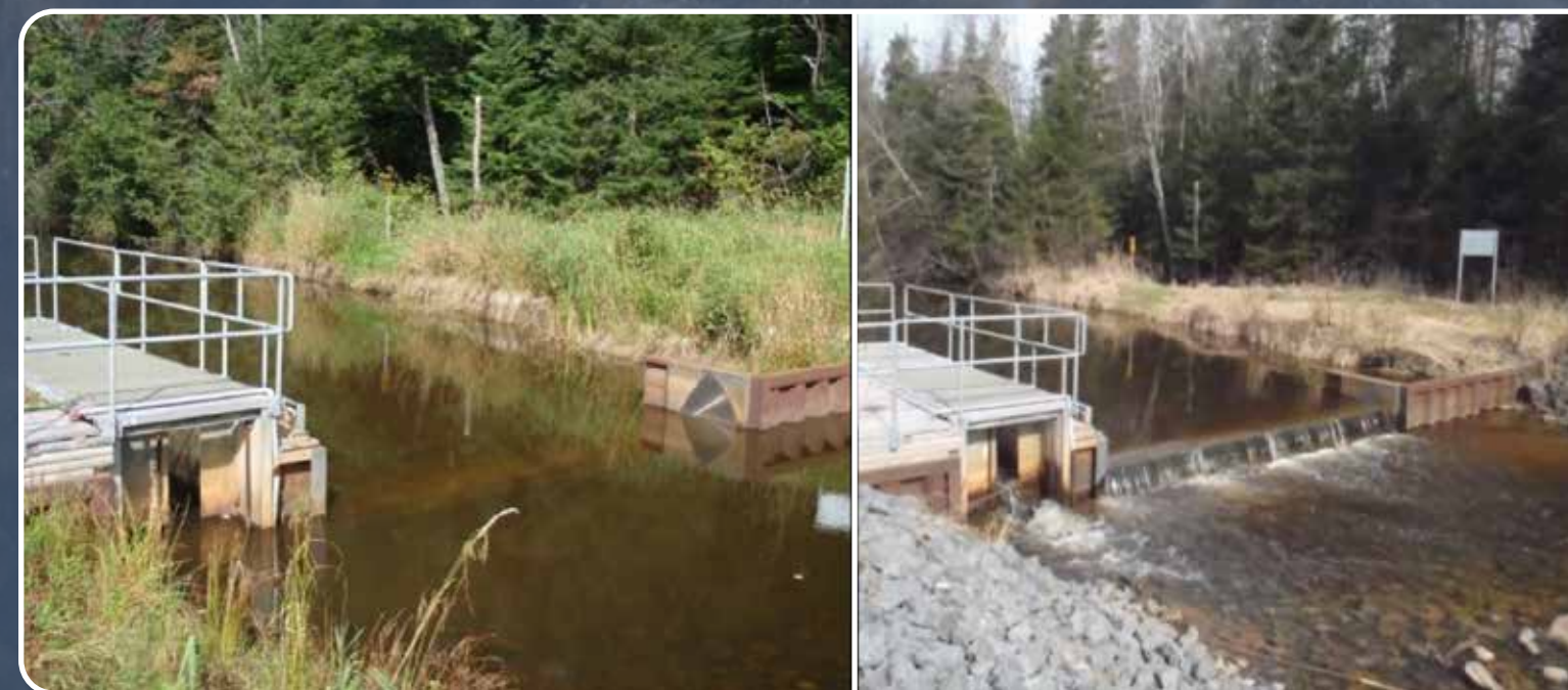
Big Carp River inflatable-crest barrier, (A) not operating with inflatable barrier down, (B) in the operating position with barrier raised (Source: Zielinski et al, 2019)
