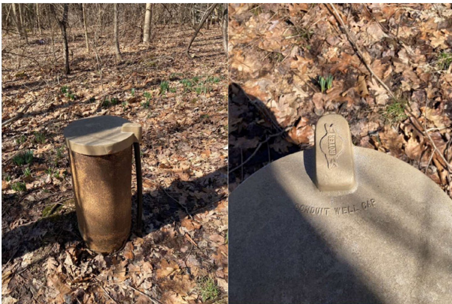
Photo 35: Steel well casing
