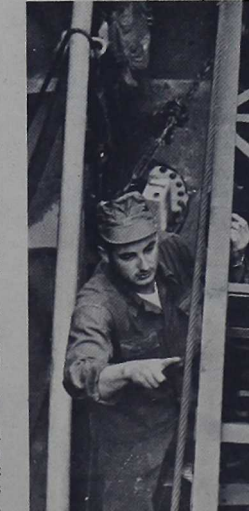
SCRAPING RUST—Lance Corporal Anthony Marchitto scrapes rust from the boom of his crane in preparation for a coat of paint.
