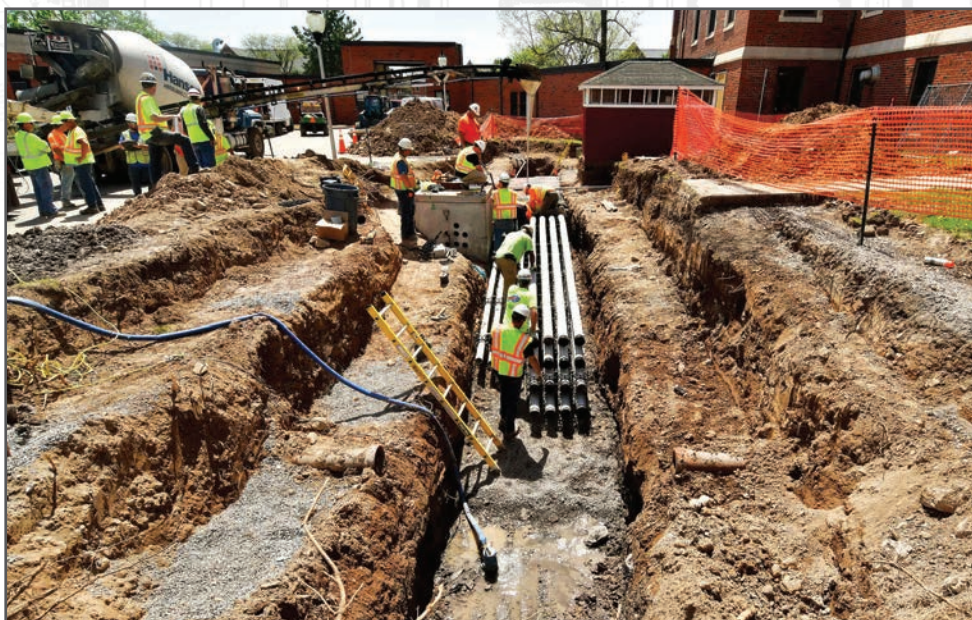
Personnel from USACE's contractor, Pike-P.J. Dick, prepare to encase electrical conduits in concrete to deliver power to the future outpatient clinic and temporary kitchen, May 18, 2018.
