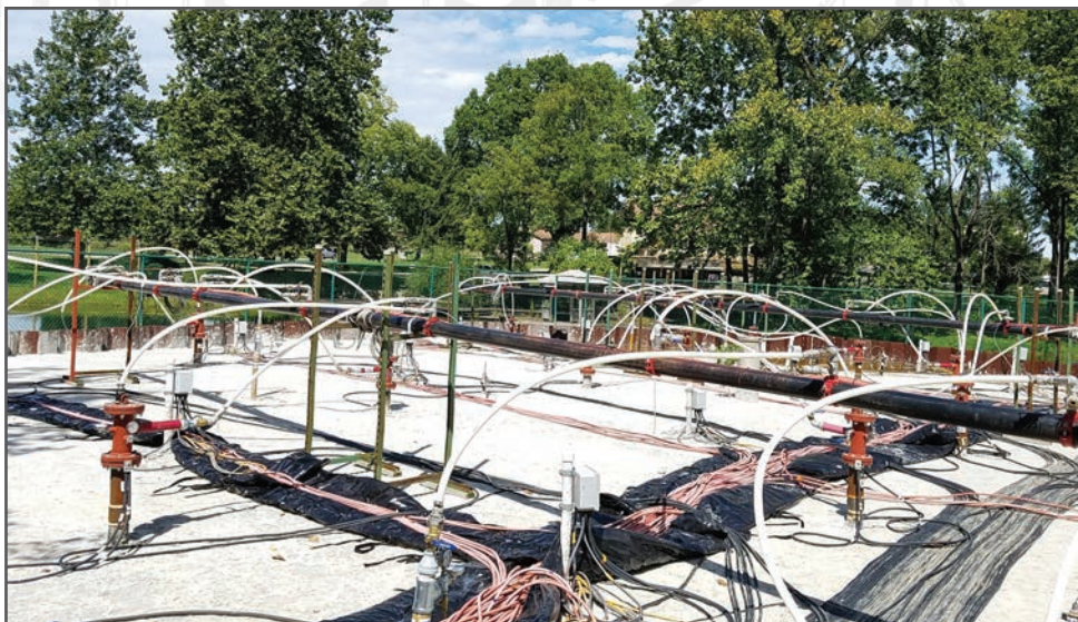
Superfund site in Zionsville, Indiana, has an electrical resistivity heating system installed to vaporize the volatile organic compounds from the impacted soil and groundwater.
