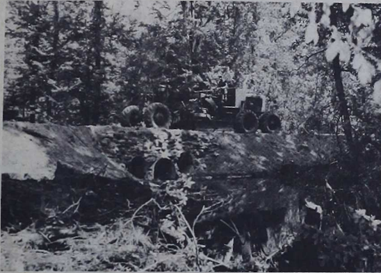
A ROAD IS "CROWNED" — A huge grader finishes up by "crowning" the new road. This process allows for water drainage. (Photo by Sgt. Carl E. Krause)
