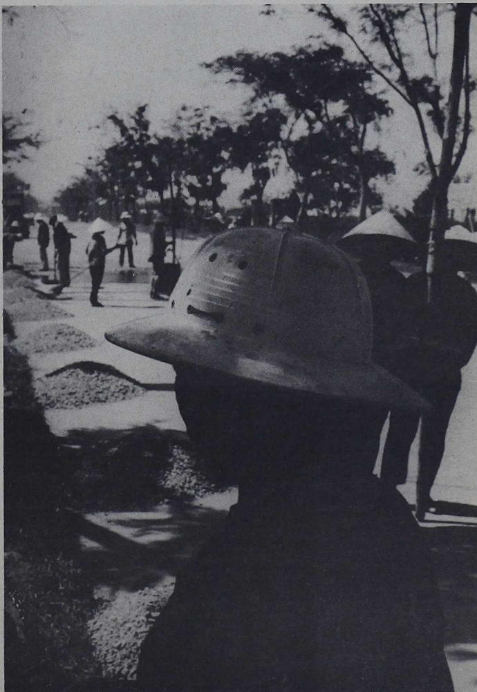
STREET REPAIR — Vietnamese Repair Trinh Ma, the main street in the walled city.
