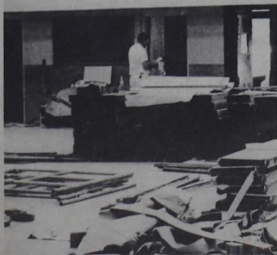
FINISHING TOUCHES — Workmen put the finishing touches on the interior of the new Post Office building on the Main Service Road here.
