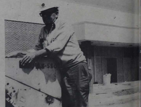
POST OFFICE — David Russell, a motor grader operator, Jacksonville, checks over his machine prior to paving driveways and parking lots at the new Post Office here. The $491,000, is scheduled to be completed this Fall.
