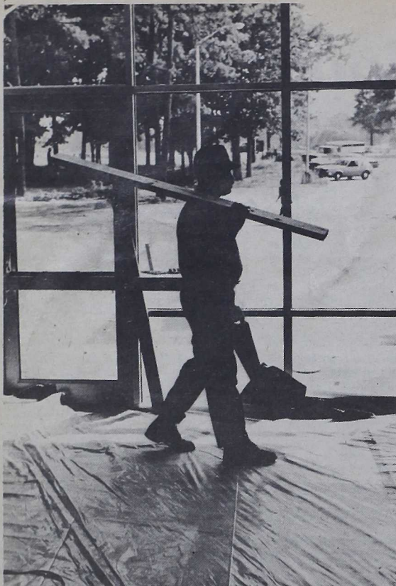
WALKING THE PLANK — Harry Lee Norman, a carpenter with the Marine Exchange, carries a piece of lumber to install on the walls of the Exchange Service building located next to the Main Exchange. Plans call for the exchange personnel to move into the new building this week.
