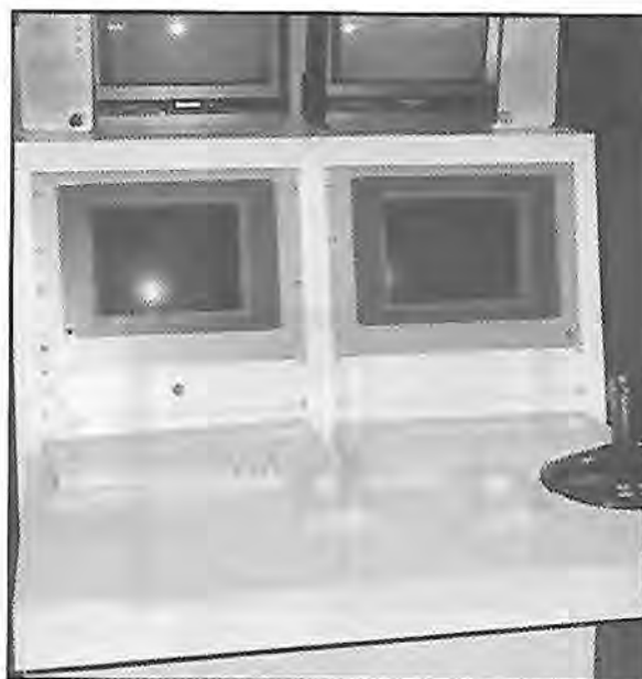
Shown here is the operator's console. The left of the two operator screens provides a macro graphics display of the robot patrol areas. The right screen can zoom in and provide a video picture if a problem is encountered. The robot will notify the operator visually and audibly of any problems. The video camera comes up with this notification so immediate action can be taken. Note: The two monitors above the operator's console are for engineering purposes only.
