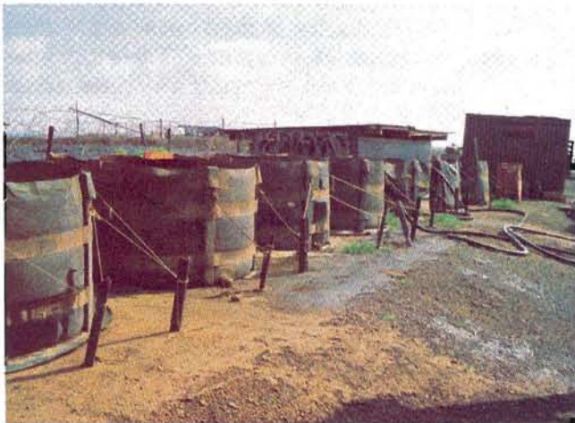
The water from this purification system was pumped to a sixteen foot tower to provide central distribution for showers, drinking, mess hall and other uses.
