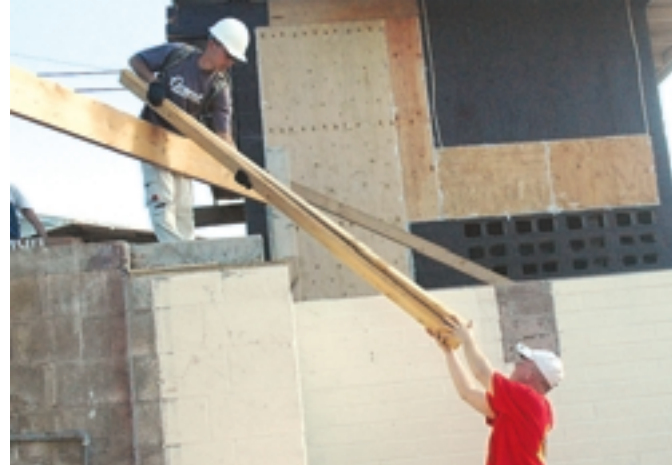
Spc. Chin Chu (top) passes two-by-fours down to Pfc. Craig Stolte. Soldiers from 82nd Engineers scrubbed and drilled holes for rebar, and then leveled pillars for the home's foundation.
