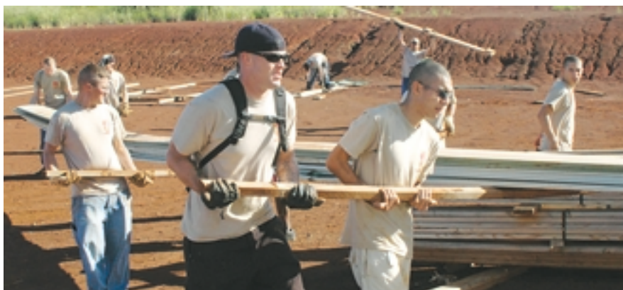
Combat engineers, squad leaders and platoon sergeants of 66th Engineer Company all jump in and provide the extensive labor required to tidy up the newly constructed Elder Care and Wellness Center at ORI.
