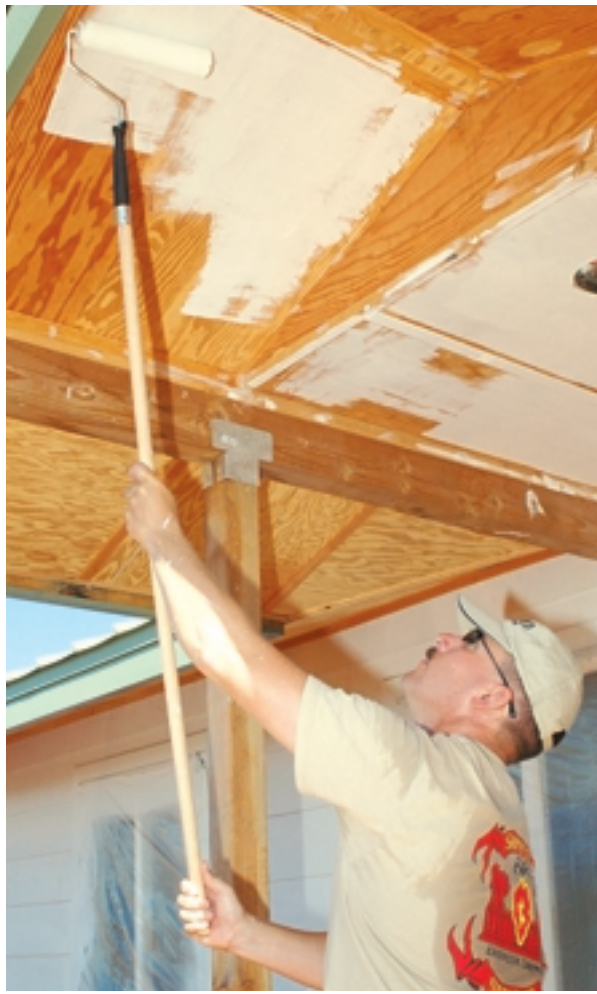
Above — Spc. Dan Jacoby, heavy equipment operator, breaks a sweat painting the roofing of a newly constructed ORI adult facility.
