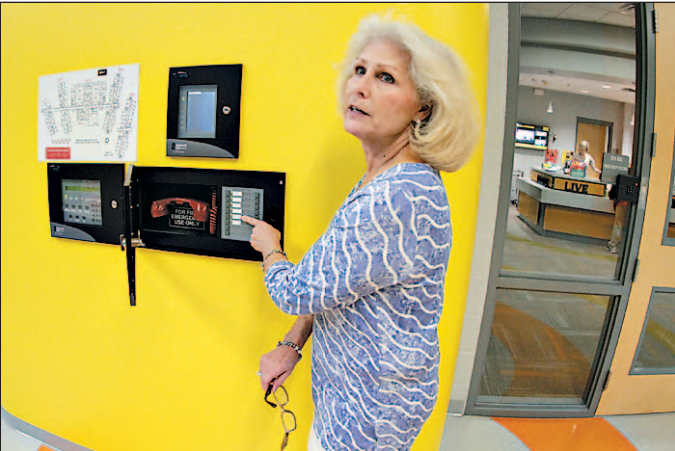
Freedom Elementary principal Mikel Shanklin shows the red phone emergency system that sends pre-programmed alert messages throughout the school.
