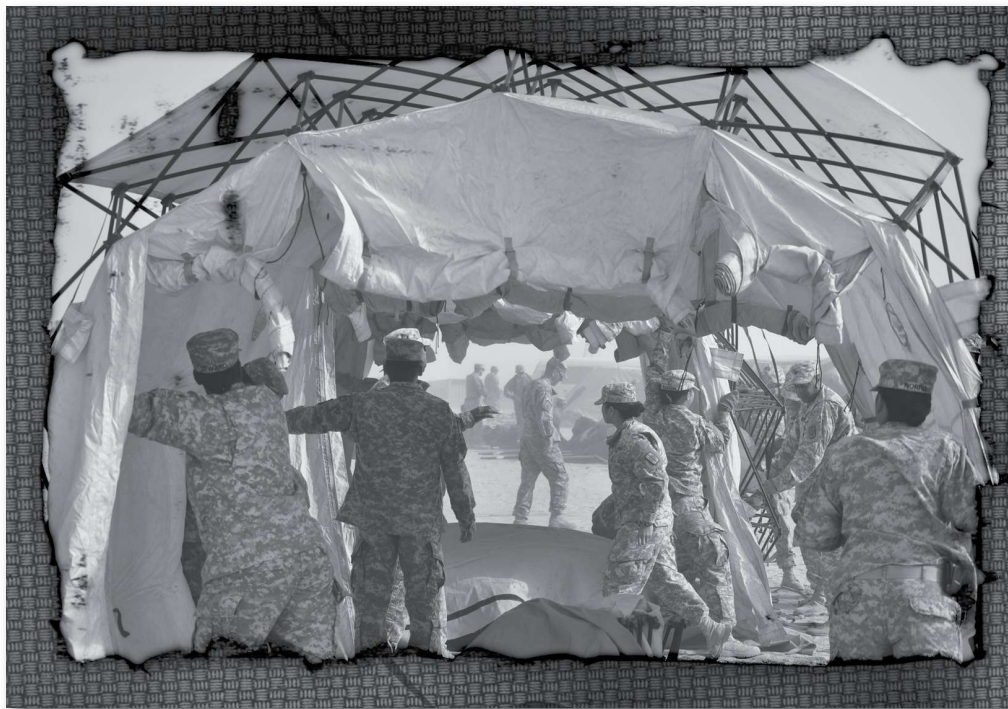
Soldiers from the 71st Chemical Company begin to set up the main tent structure for the decontamination component of the operation.
