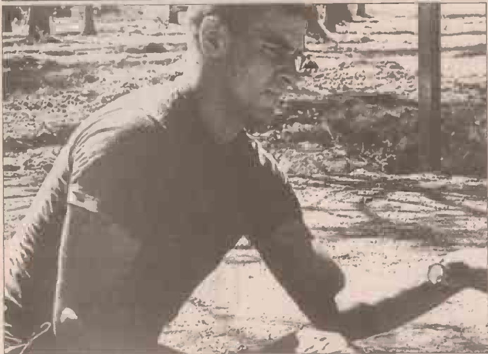
Photo by 2nd Lt. Courtney Wyckoff Pfc. Kevin J. Mitchell, 9th Engineer Support Battalion, 3rd Force Service Support Group gives the old "heave ho" to some rocks blocking a culvert during a five-week Humanitarian Assistance Operation held in Indonesia.
