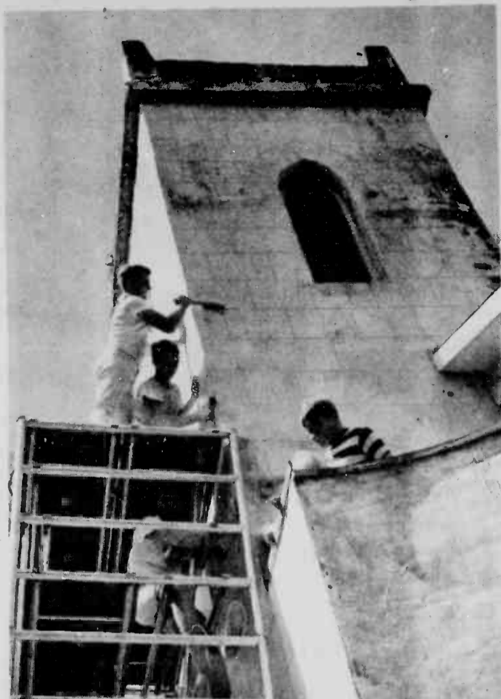
THE BEGINNING - Marines mount scaffolding to wire brush Father Damien's chapel in preparation to repainting.
