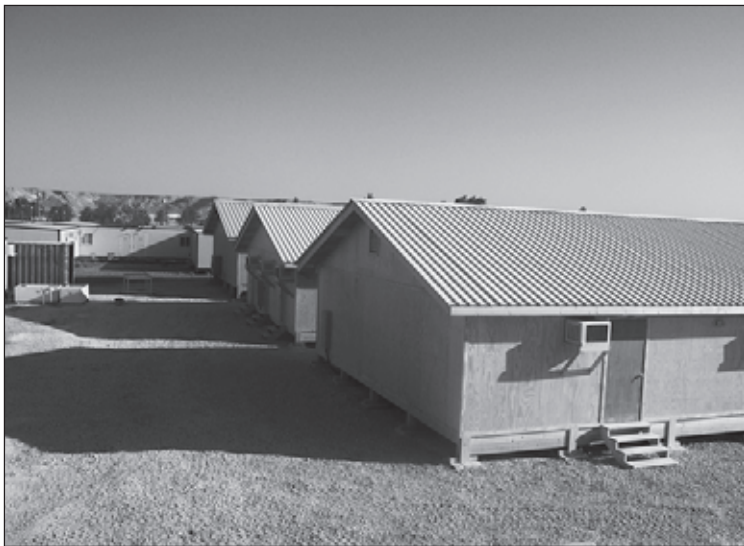
Opposite page: The frame of an exterior wall of a SWA hut awaits completion of the floor.
