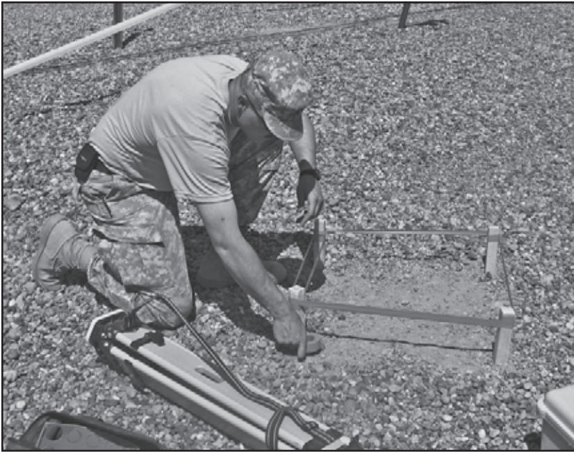
A Soldier stakes off a base station setup, which is a temporary benchmark for the survey.
