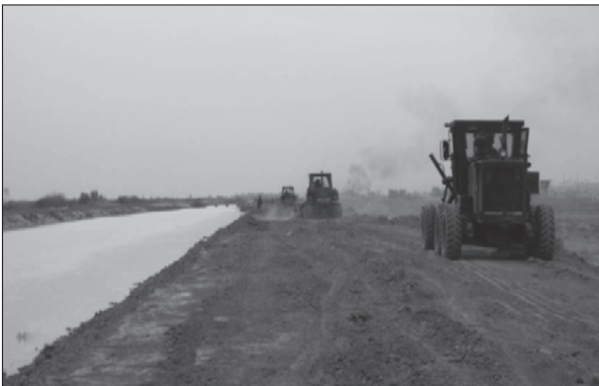
Army engineers construct a road to facilitate access to a logistics support area.
