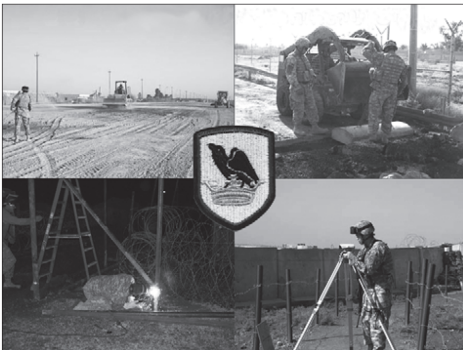
The versatile 803d Utility Detachment executes various missions: Top left – final grade for vehicle staging area; Bottom left – fence improvements for force protection; Top right – traffic speed bump emplacement; Bottom right – final survey shots for drainage and elevation.
