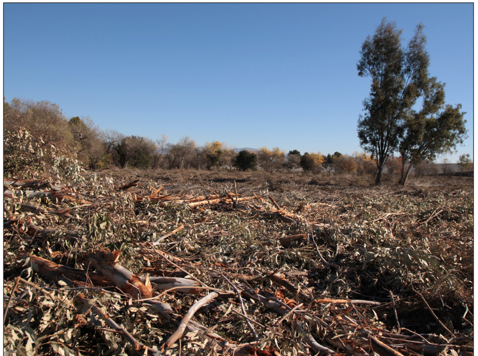
During work on the Sepulveda Basin vegetation management project that began Dec. 10, 2012, access roads (top) were opened to facilitate debris removal. Debris from a eucalyptus tree (bottom) is shown in the foreground in the Sepulveda Basin Jan. 3. In all, the Corps removed roughly 80 tons of trash and knocked down underbrush in preparation for mulching. Phase one of the five-year project is barely 25 percent complete with mulching still required, as well as selective treatment of non-native vegetation. Non-native trees and invasive species will be further identified and removed to complete phase one. (USACE photos by Dave Palmer)
