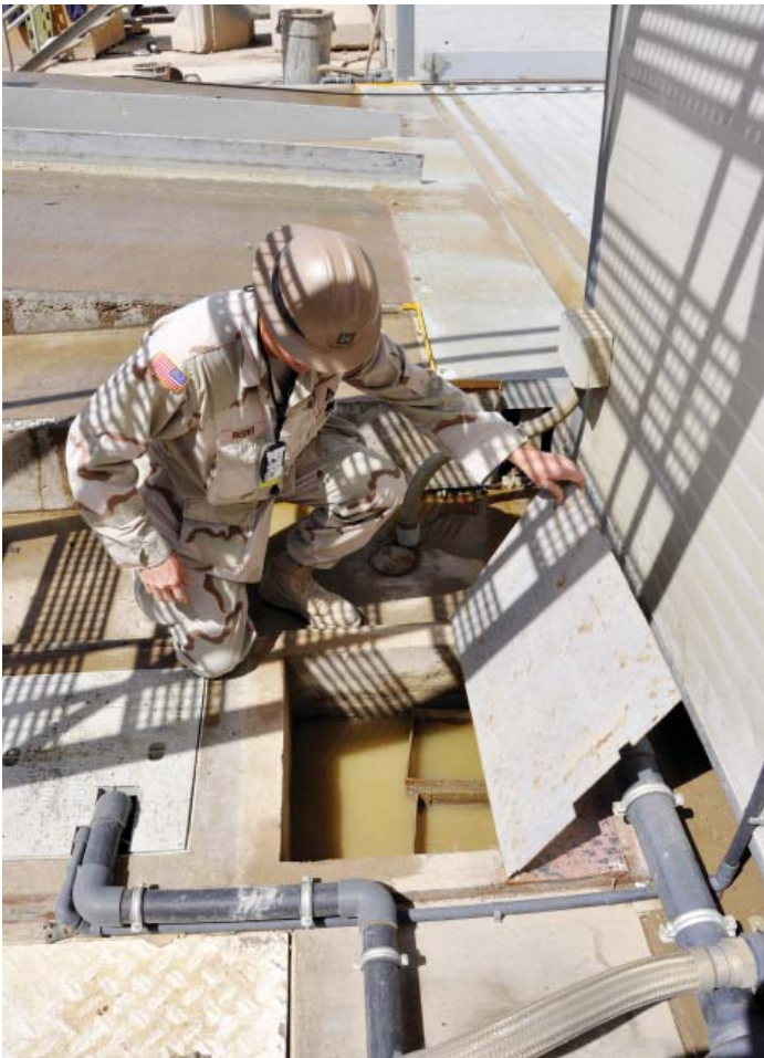
Shawn Huebner inspects the wash rack water recycling system at the Theater Vehicle Maintenance Facility on Kandahar Airfield, Afghanistan. The recycling system reuses about 80% of the water that is used for washing vehicles. (USACE Photo by Karla Marshall)
